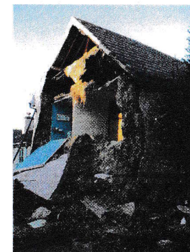
Sudden and catastrophic failure of Callarde's west gable, 8 March 2010
